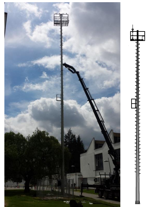
Figure 1. Installation of the 30 m high Corona current measuring mast in the campus of the Universidad Nacional de Colombia.
